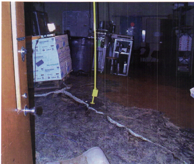
After a pipe broke underground, the floor of SLCC's print shop began to rise and buckle.
