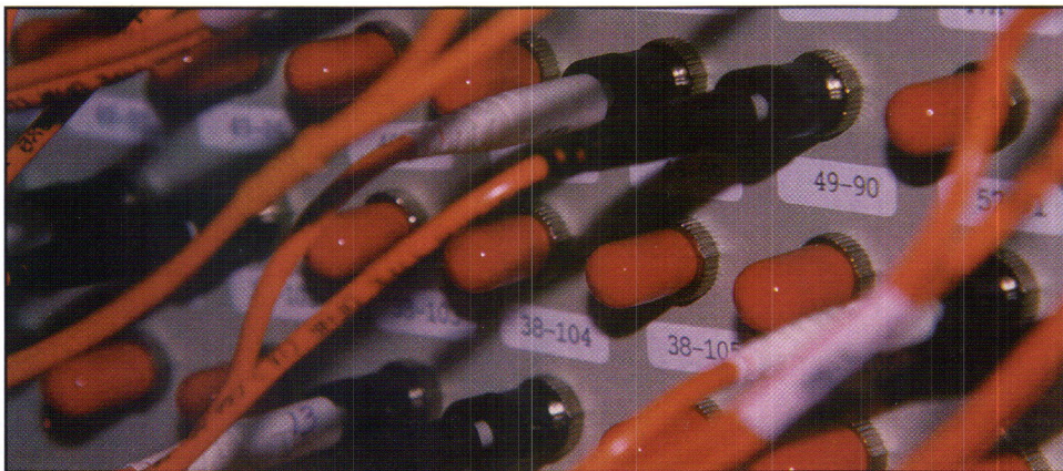
Chromatic Technologies' fiber-optic cable is terminated with Methode ST connectors to the fiber-splice boxes in the IDFs.
