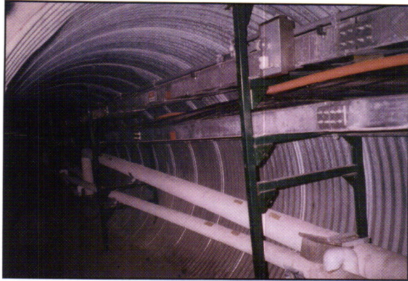
Fiber-optic cable runs through conduits in underground steam tunnels.
