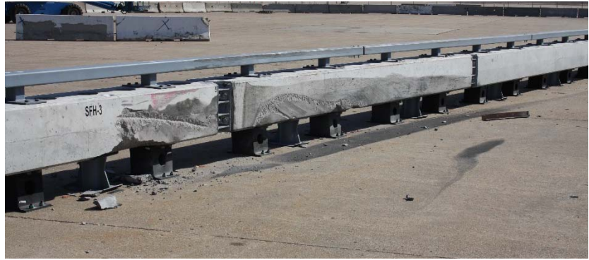
(b) System Damage
