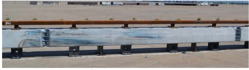
(b) System Damage
