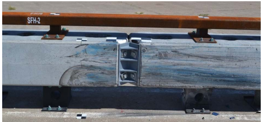
(c) System Damage
