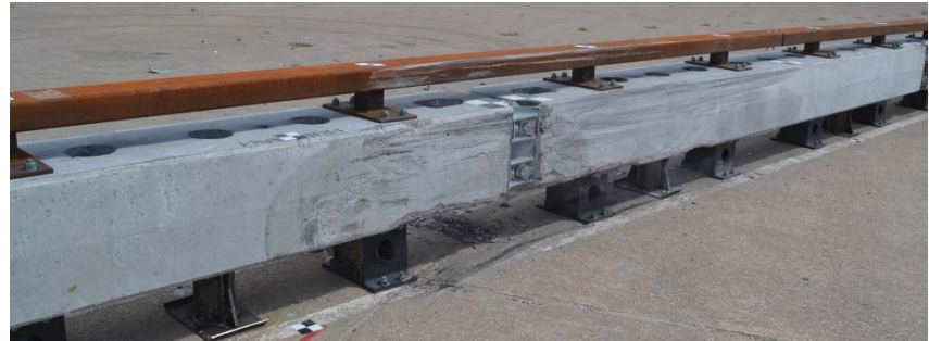
(b) System Damage
