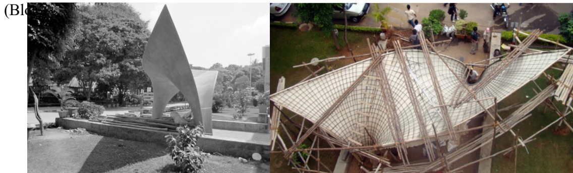
Figure 2.15 On-site fabric guide work for Bangalore shell designed by Zaha Hadid Architects, AA Visiting School in India 2011 (Block et al 2014) Retrieved from: http://www.zha-code-education.org/AA-VISITING-SCHOOL-INDIA-DELHI-JULY-2013
