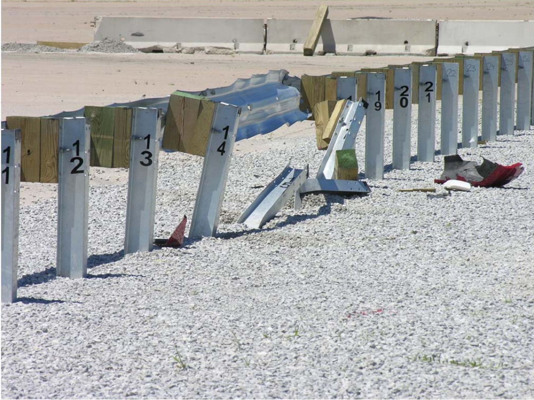
Figure 36. System Damage, Test No. MGSMRH-1
