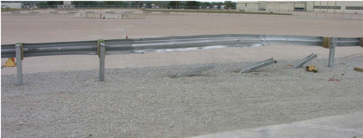
Figure 62. System Damage, Test No. MGSMRH-2
