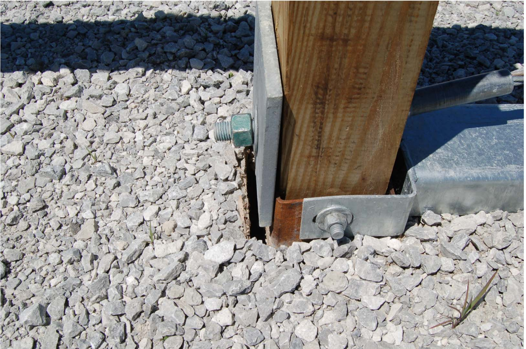
Figure 40. Soil Gap at Upstream End Anchor, Test No. MGSMRH-1
