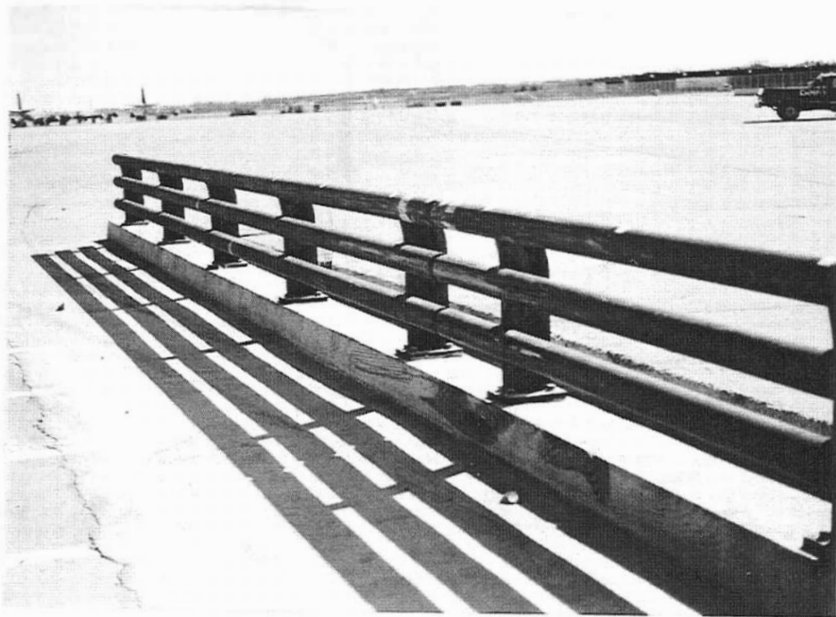
Figure 33. Bridge Rail Damage. Test GWMP-3.
