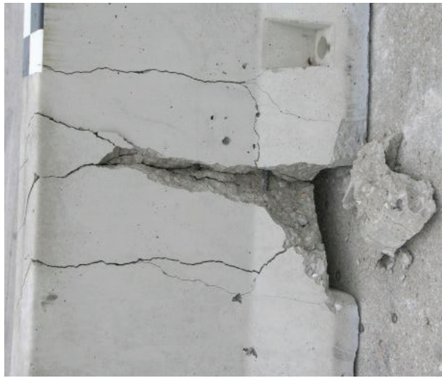
Figure 36. System Damage - Back of Barrier No. 2, Test No. TTCB-1
