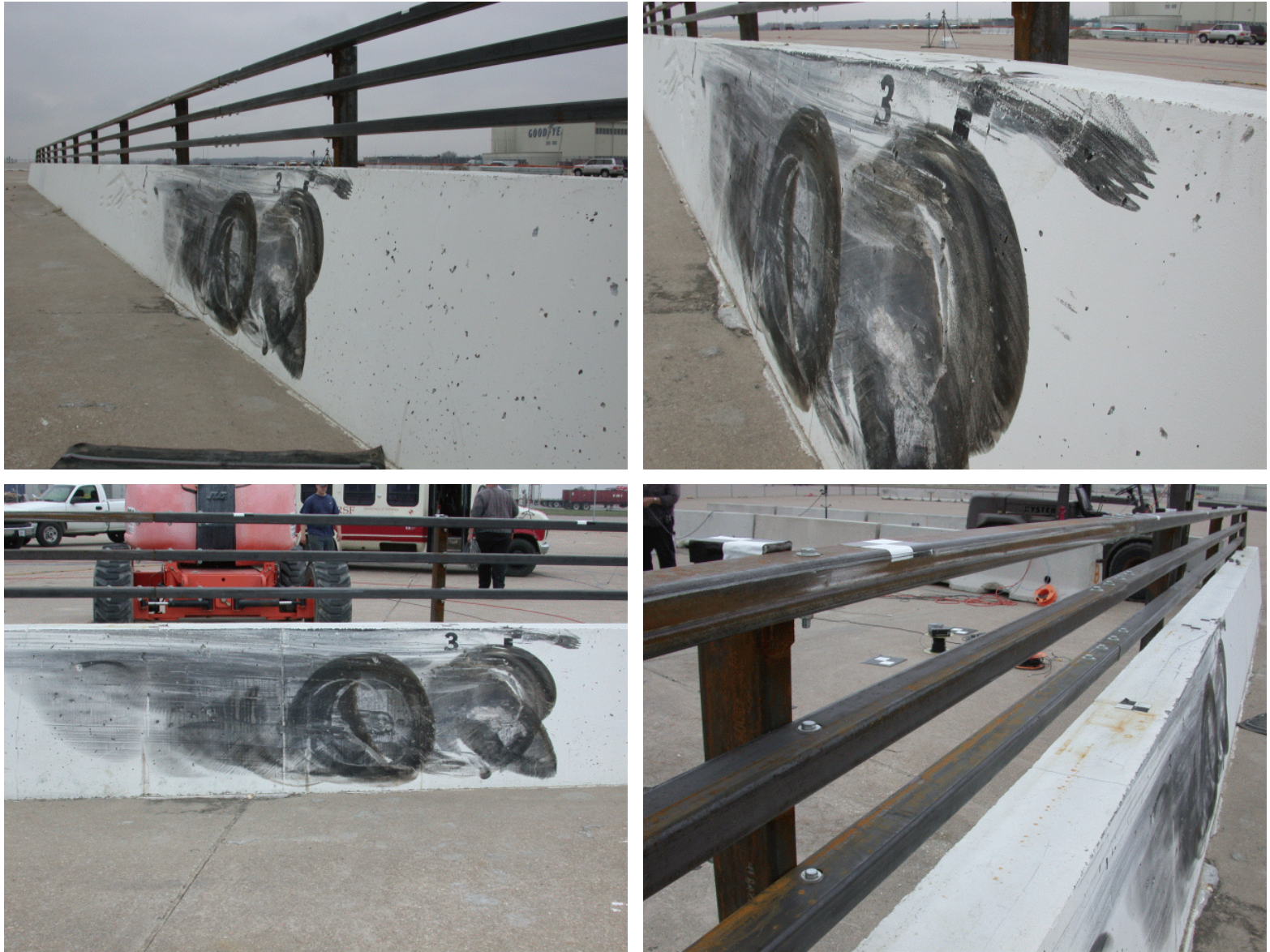
Figure 27. System Damage, Test MOBR-1
