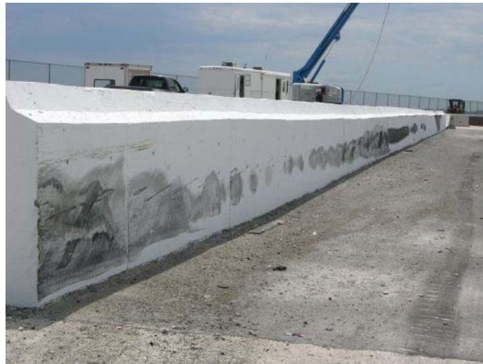
Figure 83. Tire Marks from Middle to Downstream End, Test TL5CMB-2
