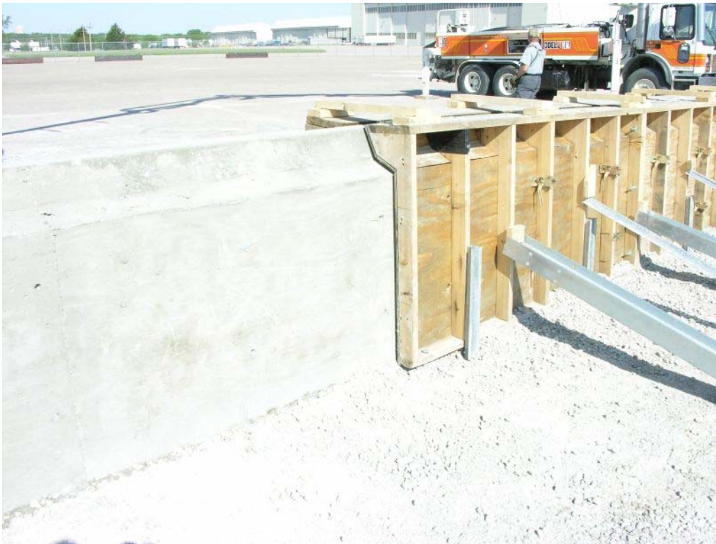
Figure 59. TL-5 Median Barrier Construction – Cold Joint
