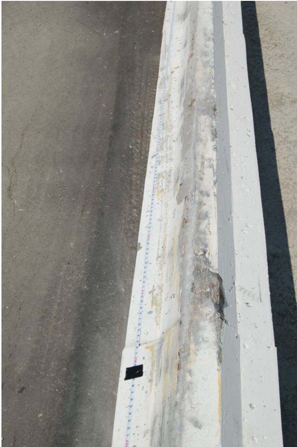
Figure 81. Barrier Damage to Top Protrusion, Test TL5CMB-2
