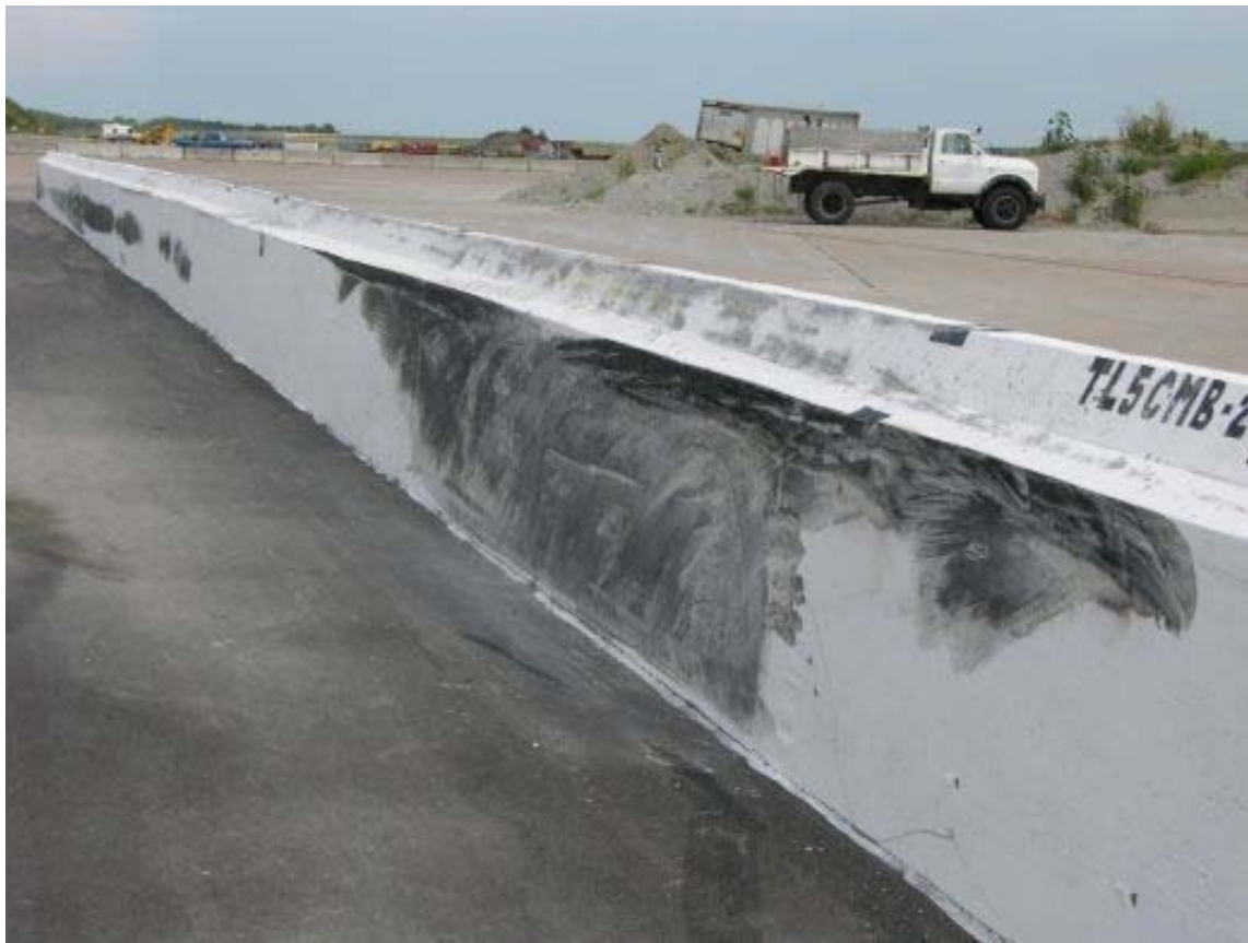
Figure 73. Barrier Damage, Test TL5CMB-2
