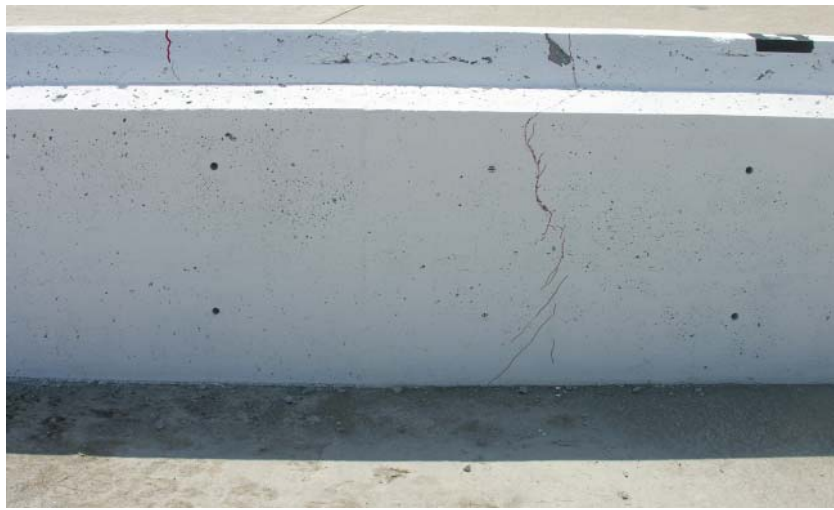
Figure 74. Barrier Cracks Upstream of Impact, Test TL5CMB-2
