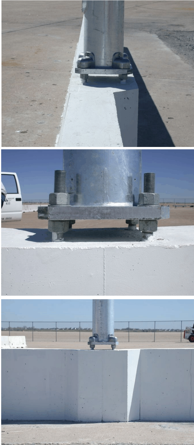
Figure 11. Luminaire Pole Attached to Single-Slope Concrete Barrier, Connection Details for Test Nos. ZOI-1 and ZOI-2
