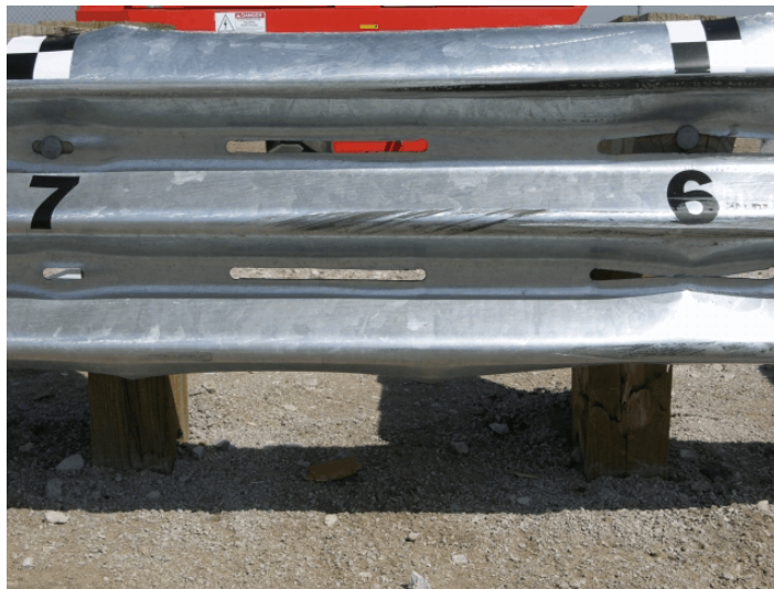
Figure 54. Rail Damage Between Post Nos. 3P through 7P, Test SR-5
