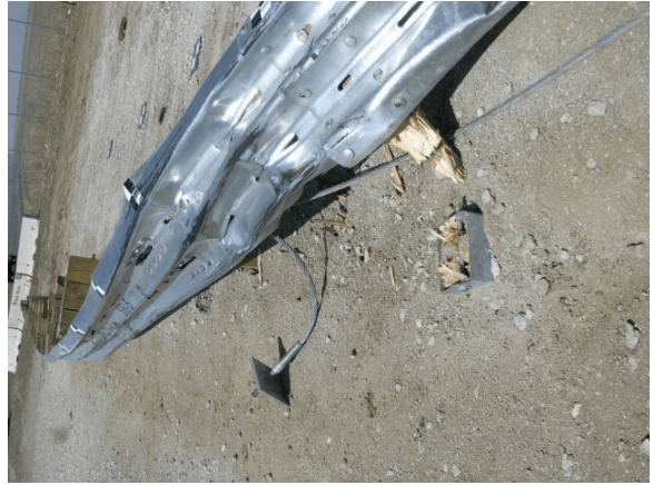
Figure 52. System Damage, Test SR-5
