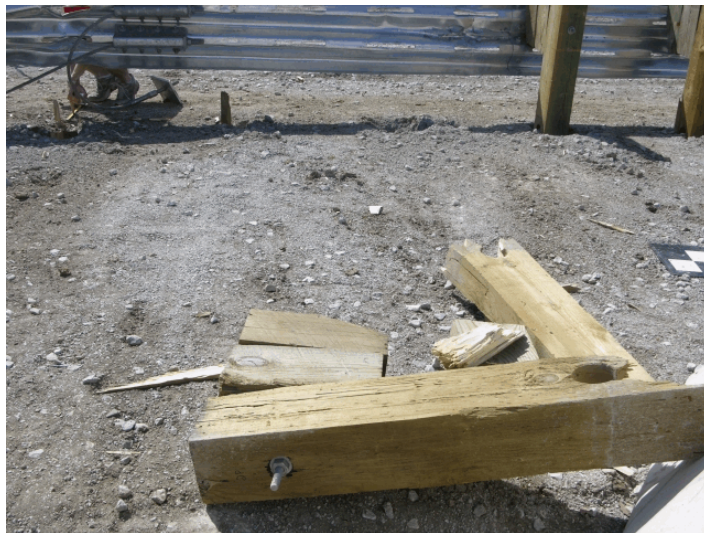
Figure 58. Post Nos. 1P through 4P Damage, Test SR-5
