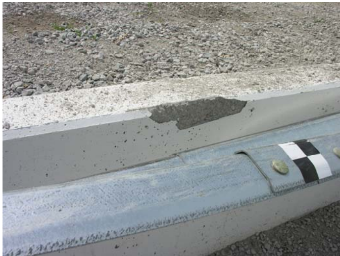
Figure 60. System Culvert Wall Damage, Test No. LSC-2
