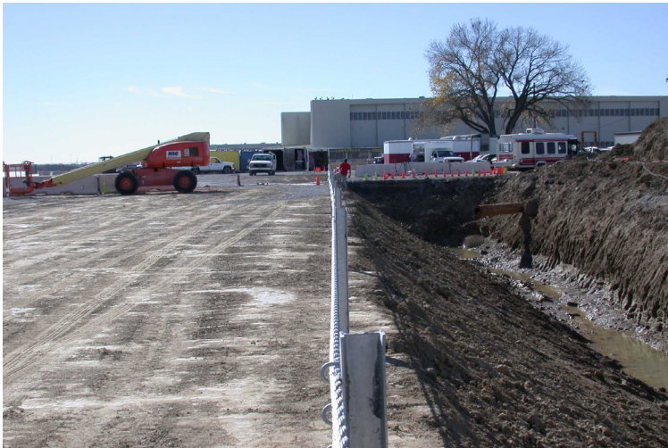
Figure 18. Three-Cable Guardrail System Adjacent to Slope
