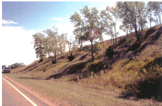
Fig. 54. Earth slump along Nebraska Highway 92 east of Arnold, Custer County. Quaternary System, Pleistocene loess. Old stabilized slide apparently controlled by vegetation roots.
