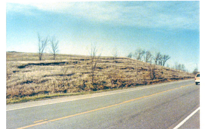
Fig. 47. Earth slump along U.S. Highway 34, six miles east of Seward, Seward County. Quaternary System, Holocene Series, Pleistocene loess overlaying glacial deposits. Recurring slide first noted in the 1960s. Majority of trees remained upright moving as a unit with slide materials.
