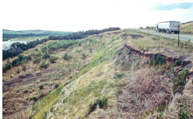
Fig. 23. Rock slump south of Niobrara. Same site as Fig. 21. Showing the slide movement along Nebraska Highway 14. Truck for scale. Road continued to move and drop so drastically that it took over 11 ft of asphalt overlays to keep road open during construction of a new third road around the slide area.
