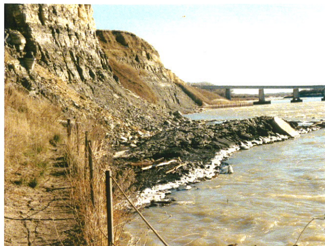
Fig. 20. Pierre Shale slump at Spencer Dam site, showing toe of slide as it emerged out and into the Niobrara River. View is downriver with U.S. Highway 281 bridge in background, crossing the river. Two previous bridges were damaged by landslides.
