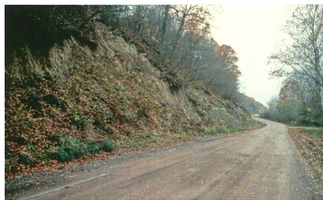
Fig. 26. Rock slump in Indian Cave State Park on a park road along the Missouri River in Richardson County. Permian System, Admire and Wabaunsee groups limestone and shale. Road was impacted by slide materials. Trees can be observed tilting above road. Missouri River bank on right side out of the picture. Road has been slightly relocated around the slide area.
