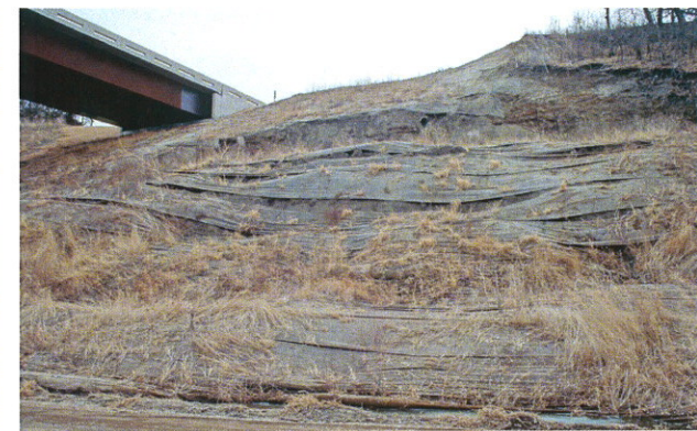
Fig. 29. Rock slump adjacent to Nebraska Highway 15 bridge over the Missouri River north of Maskell. Cretaceous System, Colorado Group, Carlile Shale Formation. Slides adjacent to bridge abutment have occurred in a newly cut slope into the shale.
