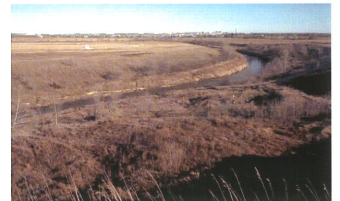
Fig. 66. Complex slide (same site as Figs. 64-65). View is from top of scarp downward to Oak Creek. Notice that slide toe has been pushed into creek causing narrowing of channel and erosion on the far bank. City of Lincoln in background.
