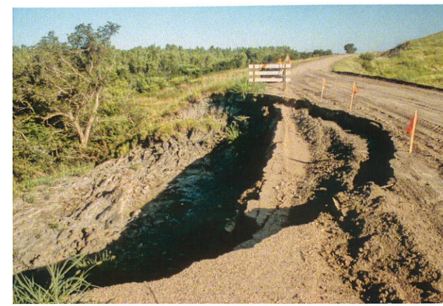
Fig. 38. Rock slump on county road north of Center, Nebraska. Cretaceous System, Montana Group, Pierre Shale Formation. Bazile Creek is to left. Similar slides often occur along this 10 mile stretch of county road.
