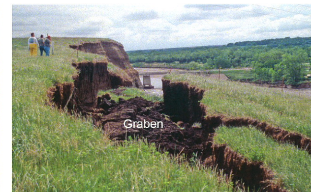
Fig. 18. Pierre Shale rock slump at Spencer Dam site showing landslide scarp and a graben. U.S. Highway 281 bridge in background. View is downriver.
