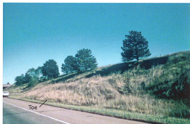
Fig. 43. Earth slump along Interstate 80 near Emerald. Same site as Fig. 42. Toe of slide nearly reached roadway. Tree roots may have curtailed further slide movements at top.
