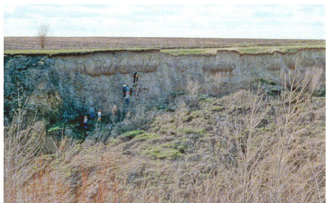
Fig. 52. Earth slump along BNSF Railroad west of Emerald, Lancaster County. Quaternary System, Pleistocene loess containing a paleosol and numerous silty clay seams. Scarp is nearly horizontal and high. Recurring Slide has closed the railroad numerous times. People for scale.
