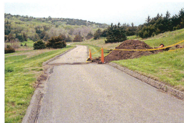
Fig. 37. Rock slump in Niobrara State Park. Cretaceous, Pierre Shale. Park road has been offset by a slow moving slide in very low slope area.
