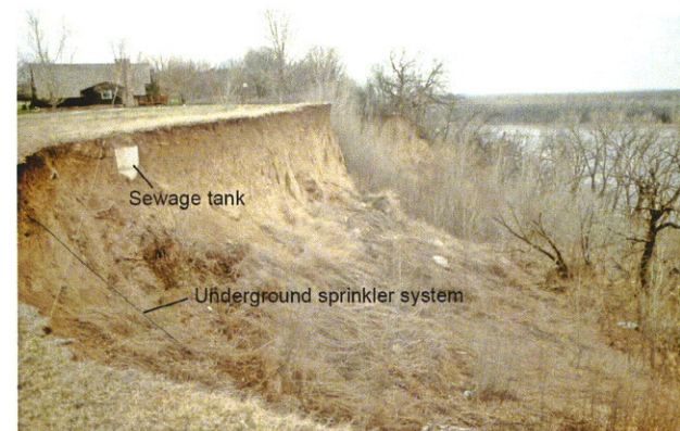
Fig. 45. Earth slump site near Fremont along Platte River bluffs, same site as Fig. 44. Sewage tank and underground sprinkler pipes are visible on left of photo.
