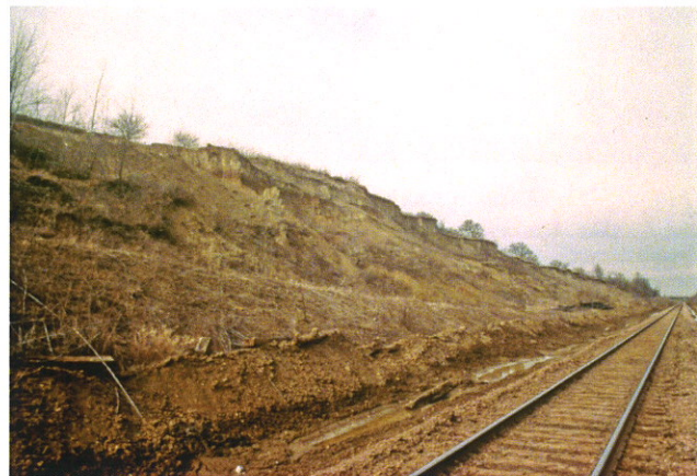
Fig. 53. Earth slump at same site as Figure 52, along BNSF Railroad. Quaternary System, Pleistocene loess. Numerous minor scarps are visible. Tracks were raised and drainage at toe was improved after slide occurred.
