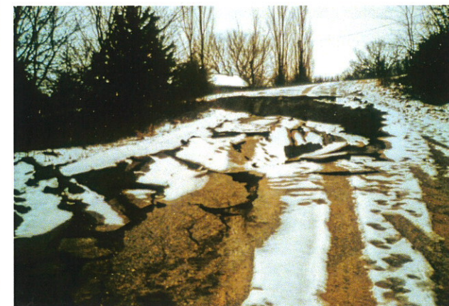
Fig. 39. Rock slump in abandoned "Devils Nest Development" in Knox County. Cretaceous System, Montana Group, Pierre Shale. Most of development was built on Pierre Shale, known landslide-prone formation. Slides impacted roads, homes, water, electrical and telephone services.
