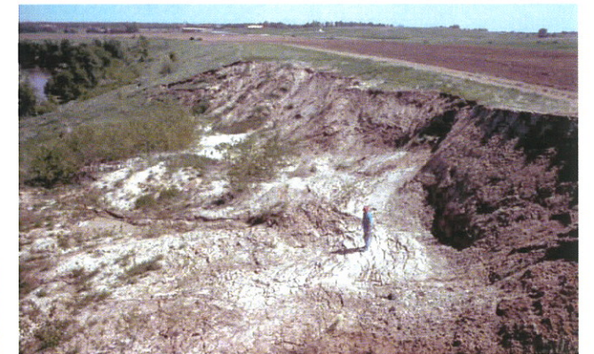
Fig. 65. Complex slide (same site as Fig. 64). View is downstream showing salts (white) that formed on displaced materials. Note person for scale.
