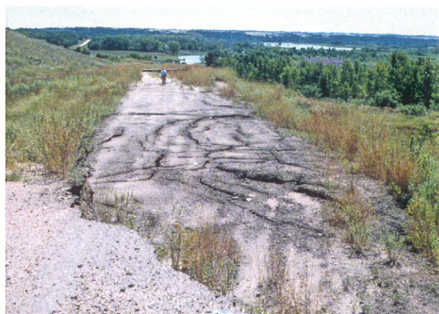
Fig. 24. Rock slump south of Niobrara. Same site as Fig. 21. Picture was taken a few years after the old road was replaced. Vertical and horizontal movement is shown. (Person in top of picture for scale).
