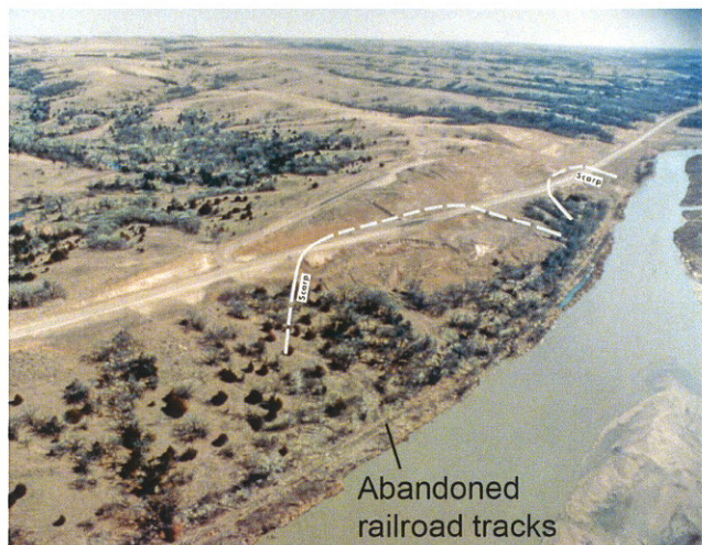
Fig. 21. On Nebraska Highway 14, 2 miles south of Niobrara, Nebraska. Large rock slump occurred in 1985, when the highway was relocated. Older road is above impacted road. In 1993 a third road was built to the left of the older road. Cretaceous System, Montana Group, Pierre Shale Formation overlain by Pleistocene sands and gravels. Two slides shown gradually became one large slide. Note abandoned railroad line located along the Niobrara River bank that also had been impacted by previous landslides.
