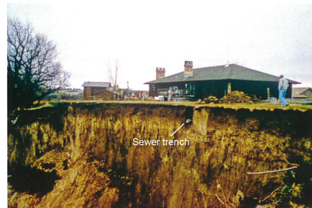
Fig. 44. Earth slump south of Fremont along the Platte River bluffs and just west of U.S. Highway 77, Saunders County. Quaternary System, Holocene Series, Pleistocene Loess underlain by thin seams of clay, silt, and very fine sand. Home was removed along with three other residences. Sewage laterals and underground sprinklers systems, seen in photo, are possible causes because water increased pore pressures, added weight, and lubricated slides.
