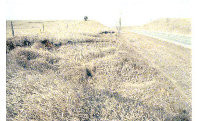
Fig. 48. Earth slump along Nebraska Highway 35 east of Hoskins, Wayne County. Quaternary System, Pleistocene loess.
