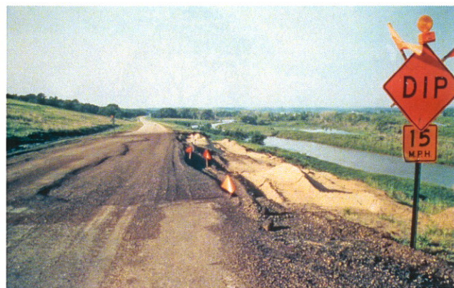
Fig. 22. Rock slump south of Niobrara involving Pierre Shale. Same site as Fig. 21. Shortly after road was constructed two small slides developed along Niobrara River valley side (right). Picture shows overnight settlement of the asphalt overlay.
