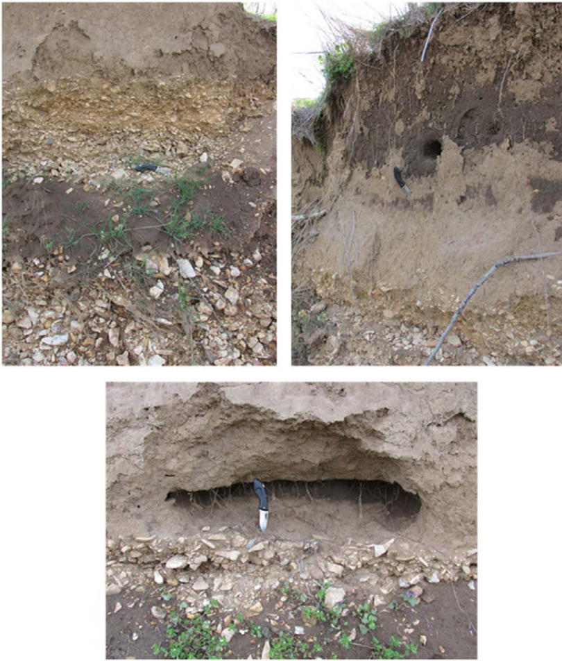
Fig. 1. Streambank at the Barren Fork Creek field site including the bank profile (top left), a megapore (top right), and a seepage undercut (bottom). Note the sloughed material at the bottom of each picture from recent bank failures. These complex alluvial deposits include both clean gravel lenses associated with rapid flow and transport (top left) and fine gravel lenses that can cause lateral flow and seepage erosion (bottom).
