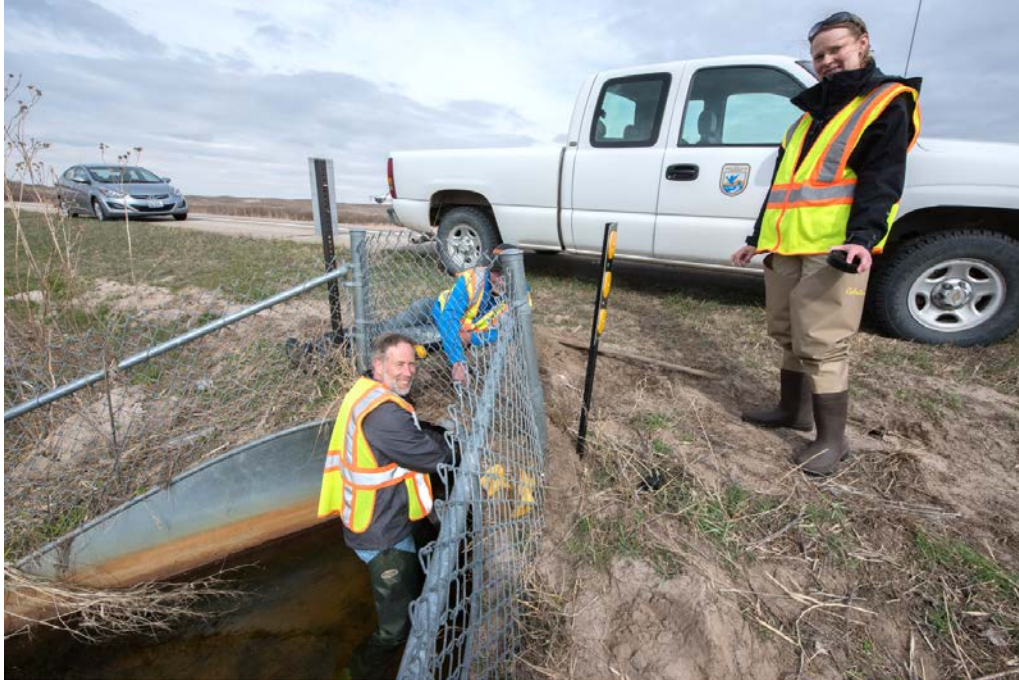
Figure 3: Installing a camera at a culvert (Sweetwater) along US Hwy 83 through Valentine National Wildlife Refuge, Nebraska.
