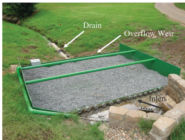
Fig. 1. Picture of the phosphorus (P) removal structure with runoff inlets, drain for treated water, and overflow weir. The P sorption material in the structure is 2712 kg of 6.3- to 11-mm-diameter steel slag.
