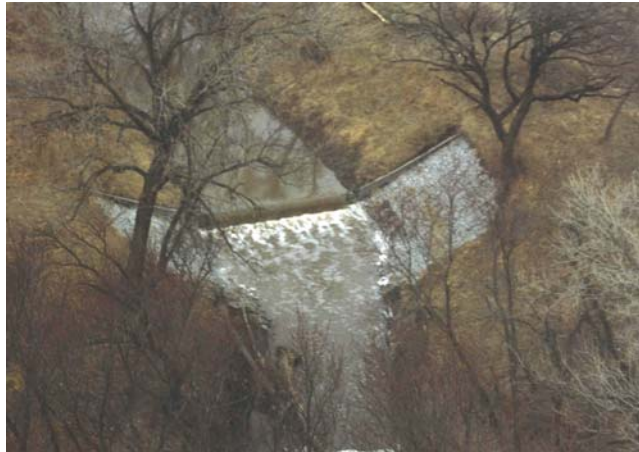
Figure 34. Grade-control structure on Big Indian Creek between Gage County Road (BBR-11) and US77 (BBR-12).
