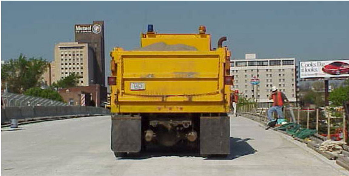
Figure C-3: Longitudinal view of Phase II lane A live load test. This view is looking West with the man at left standing near the closure region. Men at the right are positioning the truck
