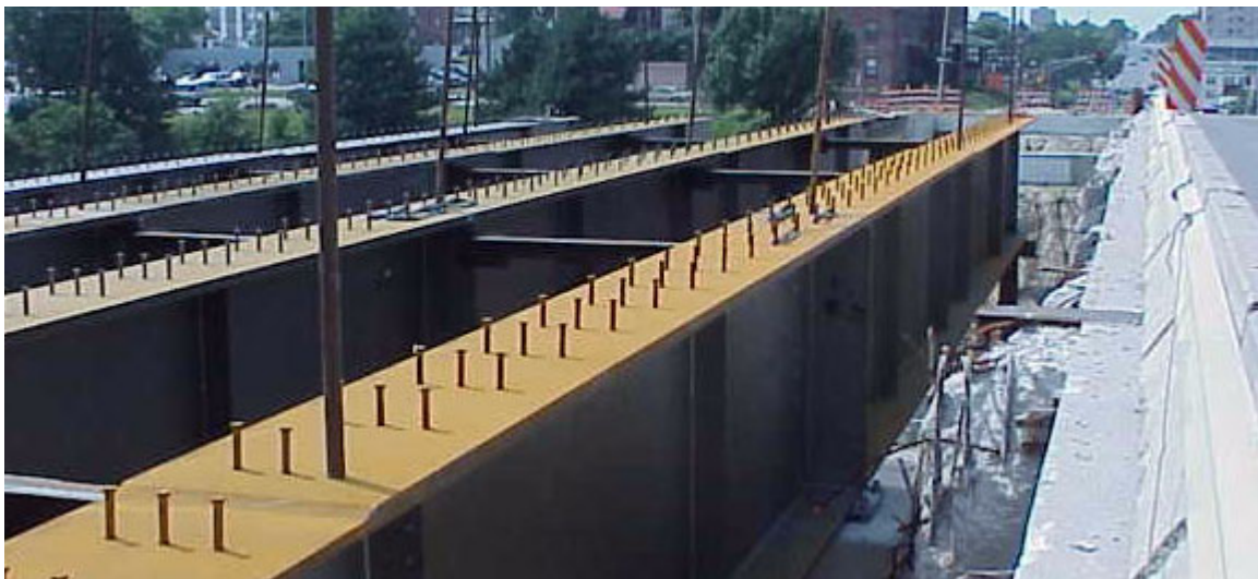
Figure 3-4: Shear Studs on the top flange. Picture is taken looking West. From right to left are Girders E, G, H, and J during erection for Phase I.
