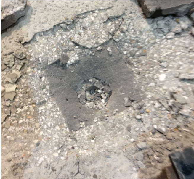
Figure 5.24: Pullout failure mode
