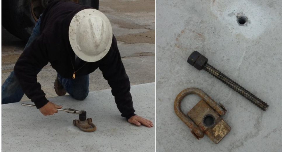
Figure 6.7: The coil rod with nuts and swivel plates used for panel lifting
