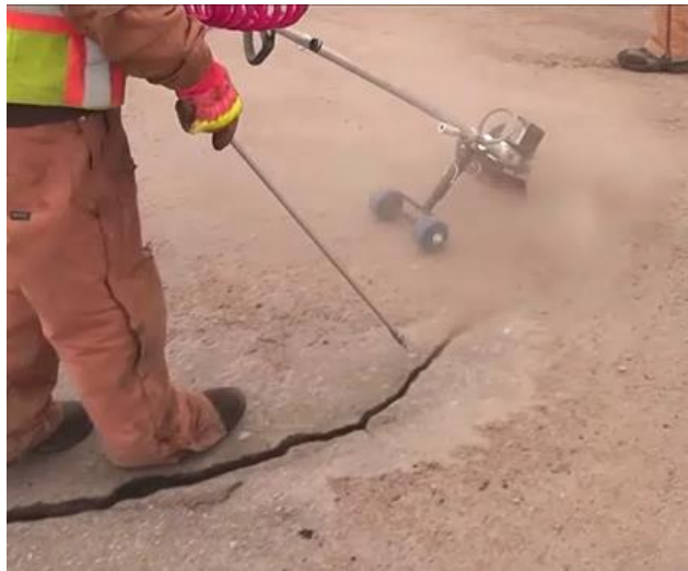
Figure 2.6 Using a detachable air wand for pavement surface cleaning by an NDOR crew
