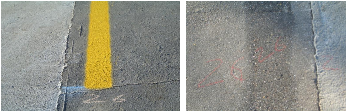
Figure 6.3. Asphalt pavement condition before (left) and after (right) 10 mils water-based paint has been removed by water blasting
