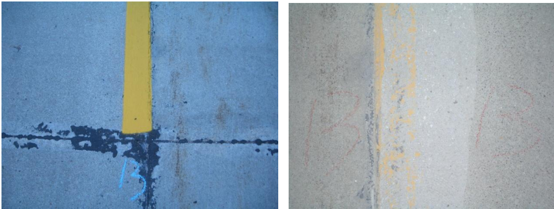
Figure 6.10. Concrete pavement condition before (left) and after (right) paint has been removed by grinding
