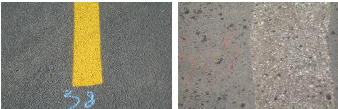
Figure 6.15. Concrete pavement condition before (left) and after (right) 12 mils paint has been removed by PCD grinder
