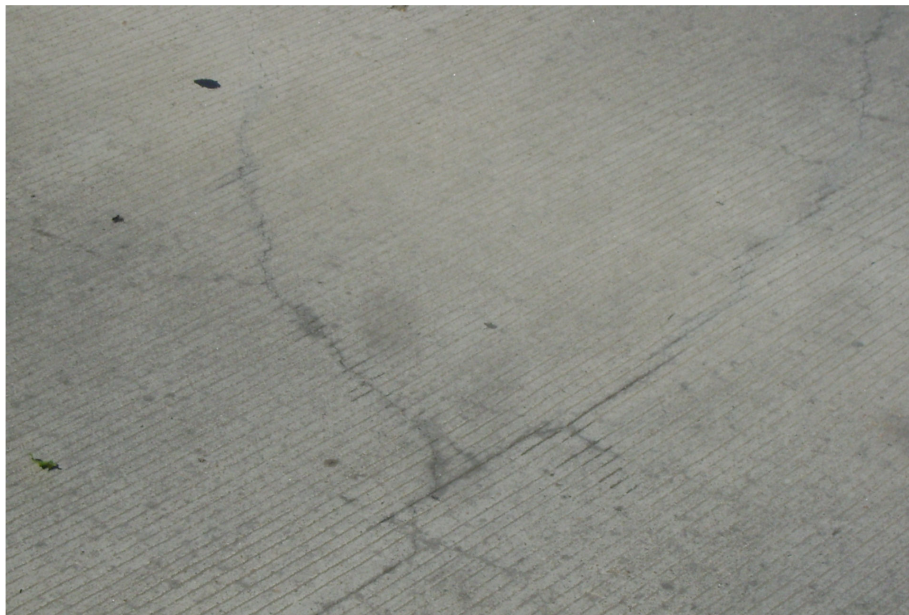
Figure A.17: Shrinkage Cracking
