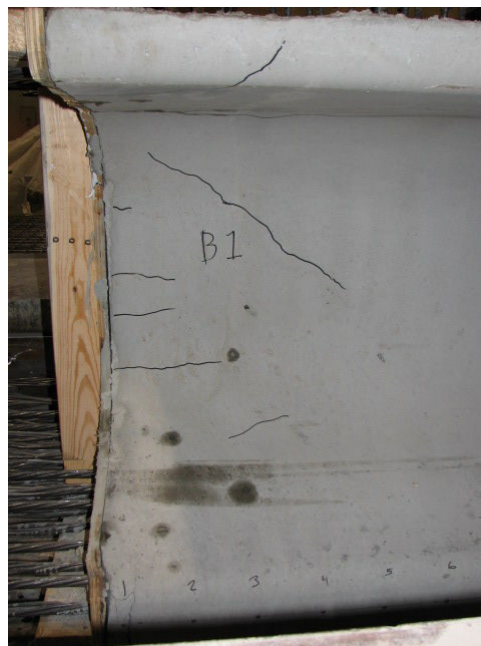
Figure 2.7.3: B1 end zone cracking
