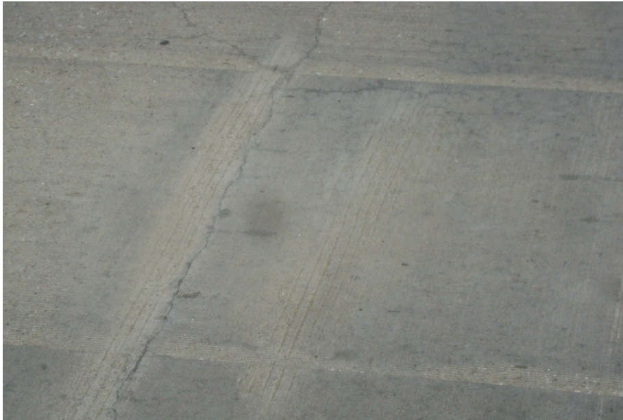
Figure A.16: Shrinkage Cracking
