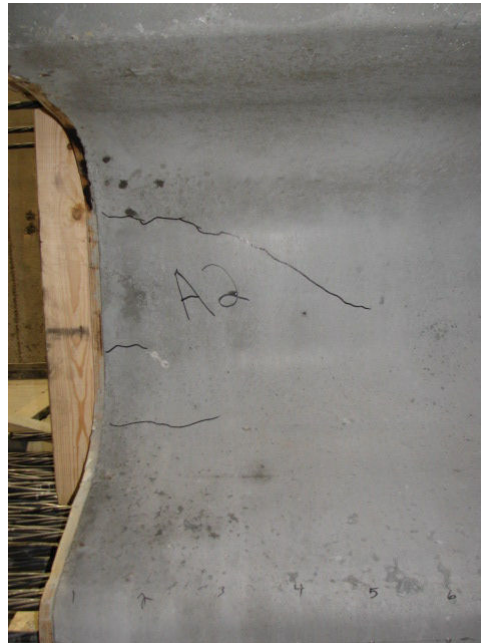
Figure 2.7.2: A2 end zone cracking
