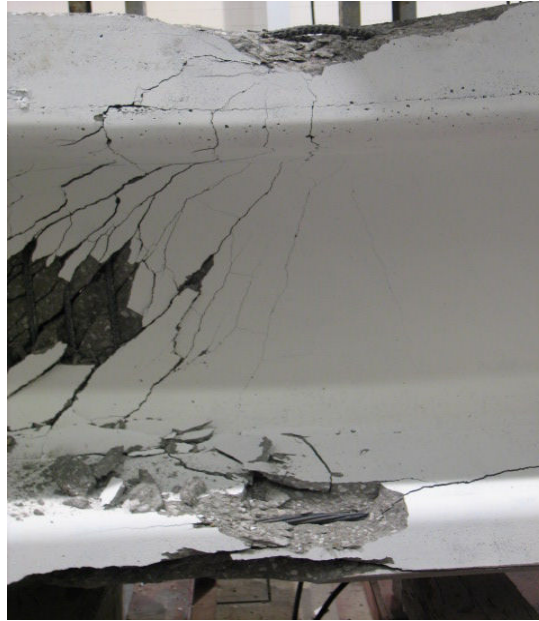
Figure 2.11.4.8: Buckling of top deck #5 bar
