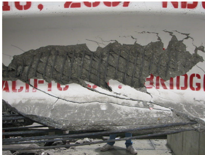
Figure 2.11.4.6: Shear cracking in web and split flange
