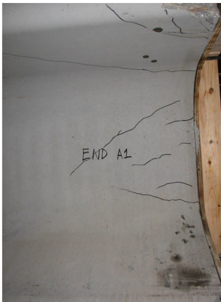
Figure 2.7.1: A1 end zone cracking
