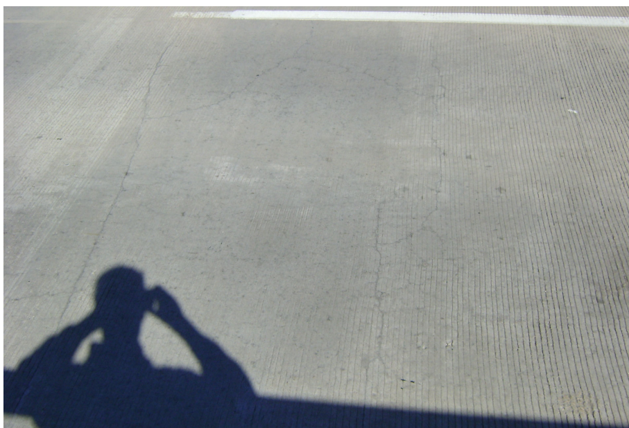
Figure A.15: Shrinkage Cracking
