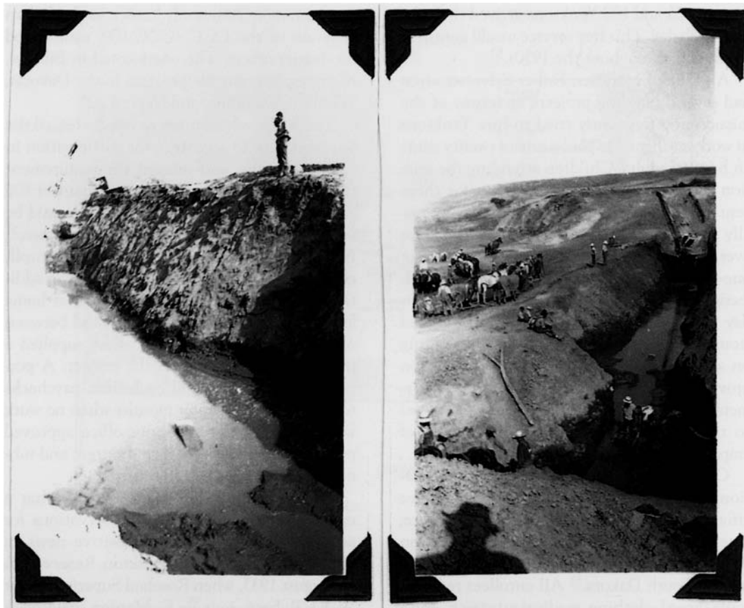
FIG. 4. (left) Problems Arise on Dam Number 75. Water and mud slowed progress and had to be removed. (right) Work on Dam Number 75. Crews and a mechanical shovel create a trench to prevent future seepage. Source: Report on Dam Number 75, Box 4, Narrative and Pictorial Reports, Records of the CCC-ID, RG 75, National Archives.
