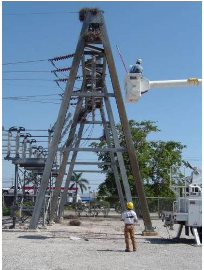
Figure 4. At electric utility substations, such as this A-frame structure in south Florida, monk parakeet nests are an ongoing maintenance concern.
