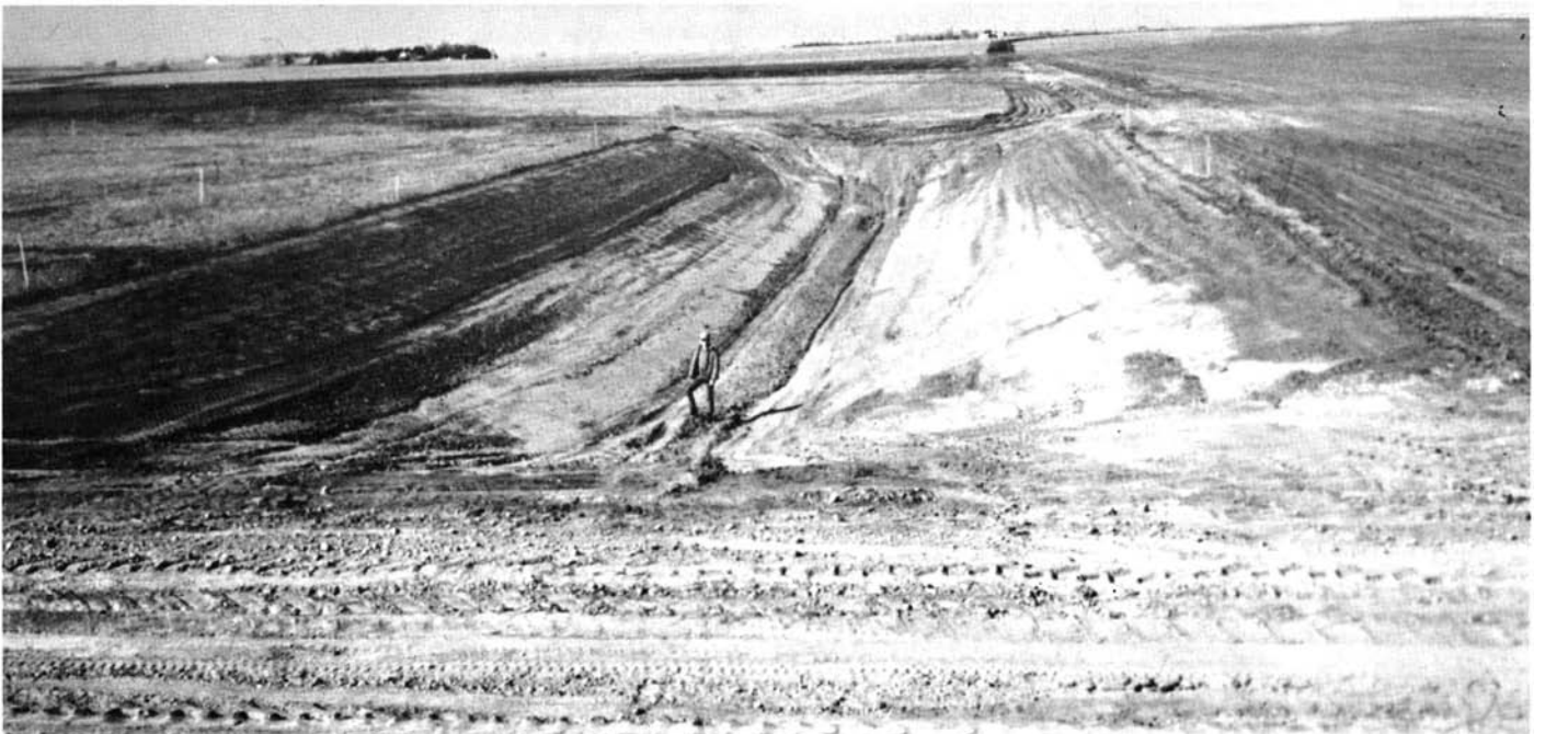
Dugout excavation (20,000 cubic yards) showing method of leveling spoil with subsequent destruction of rainwater basin.
