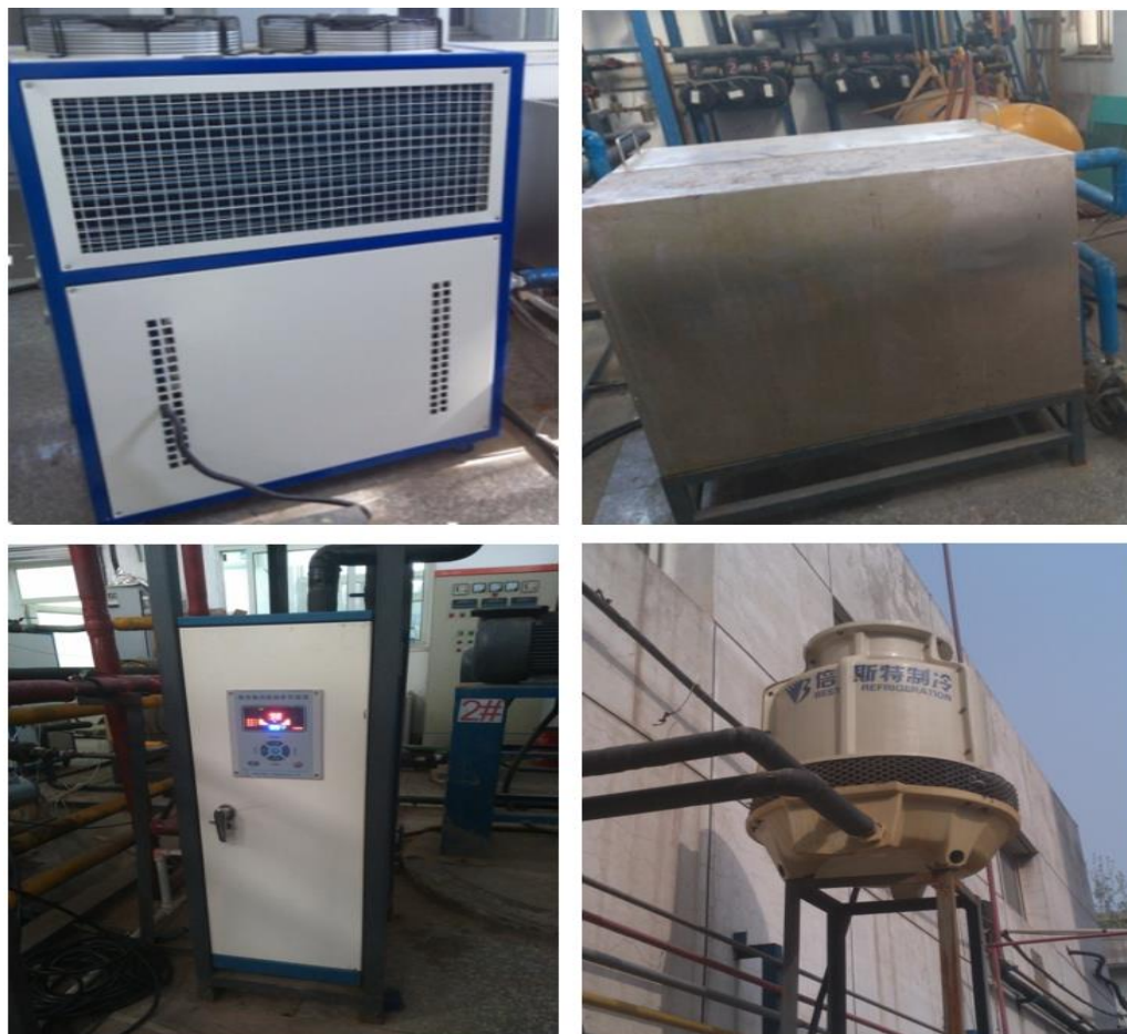
Figure 4-6. Photos of main instrument in water loop system
