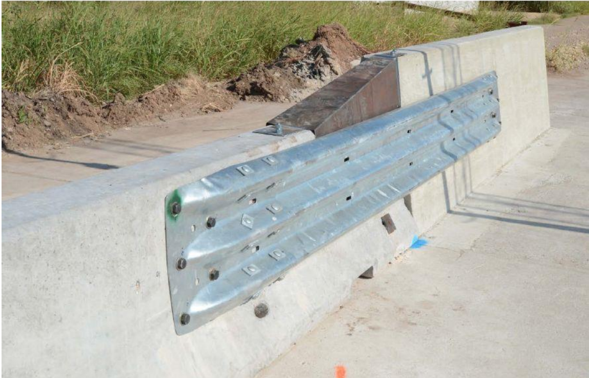
Figure 22. Free-Standing PCB to Rigid Barrier Height Transition for Roadside Applications on Concrete [46]
