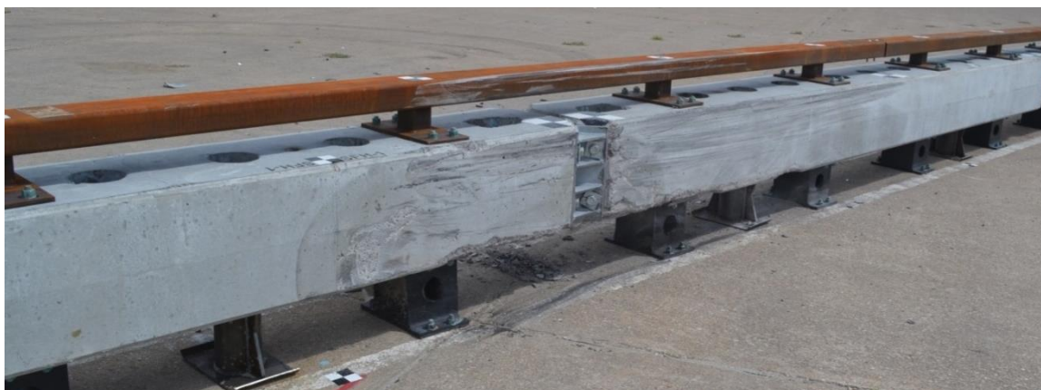
Figure 40. RESTORE Barrier Damage, Test No. SFH-1 [20-21]
