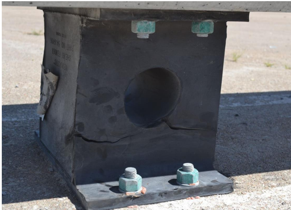
Elastomer Post Damage
