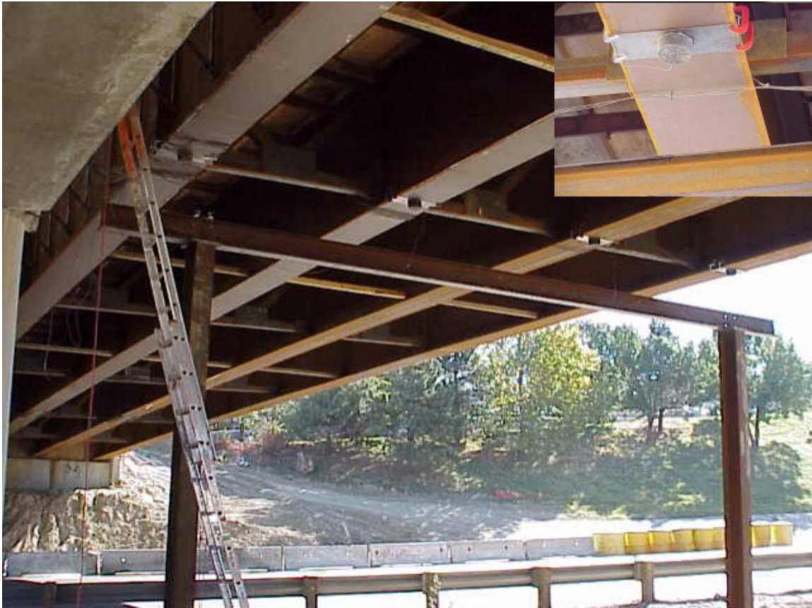
Figure B-15: Test frame used to measure deflection. Note pots mounted on the underside of girders
