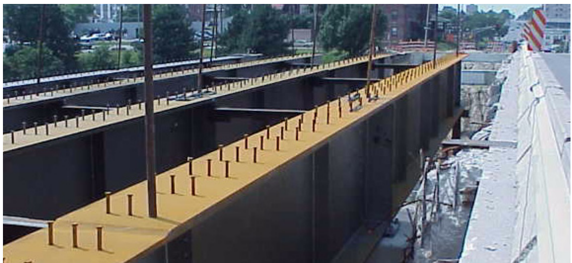
Figure 2-4: Shear Studs on the top flange. Picture is taken looking West. From right to left are Girders E, G, H, and J during erection for Phase I.
