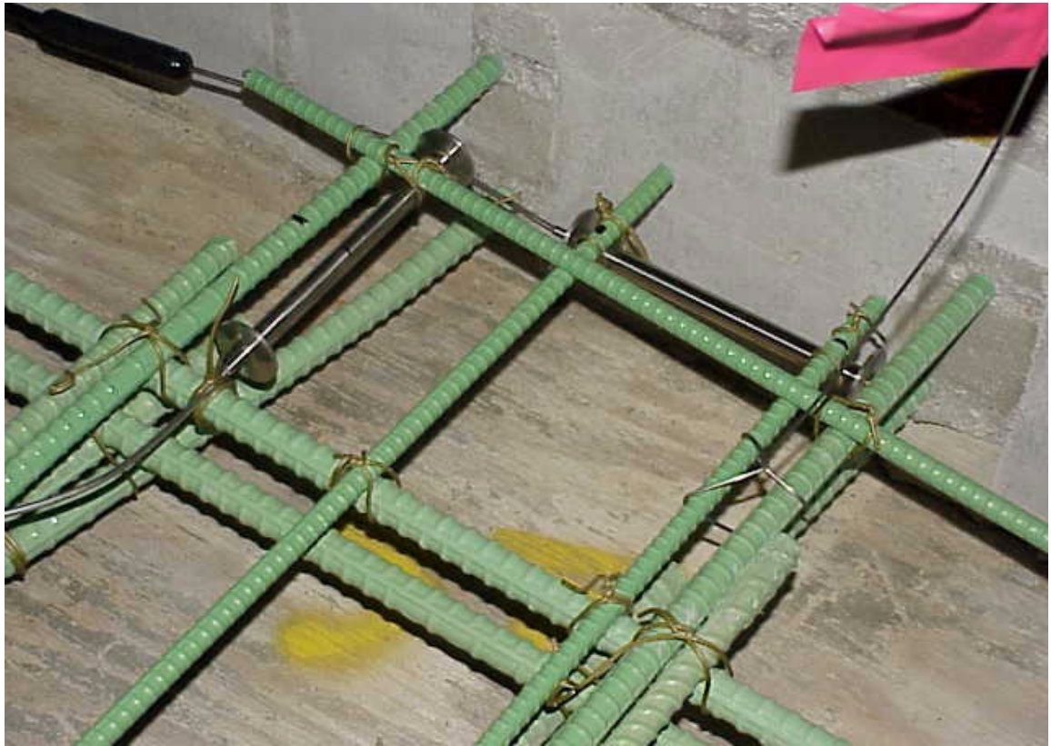
Figure 2-34: Concrete Embedment gage in place. These gages record concrete strain.
