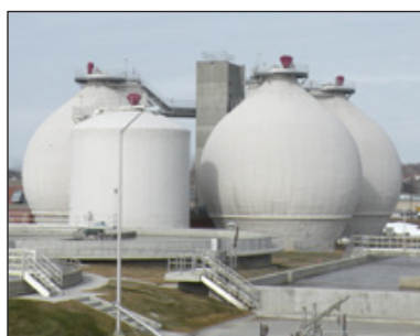
Egg-shaped anaerobic digesters at the Theresa Street Wastewater Facility break down the wastewater solids into a more stable form. This process makes biosolids suitable for use by area farmers as a fertilizer.
