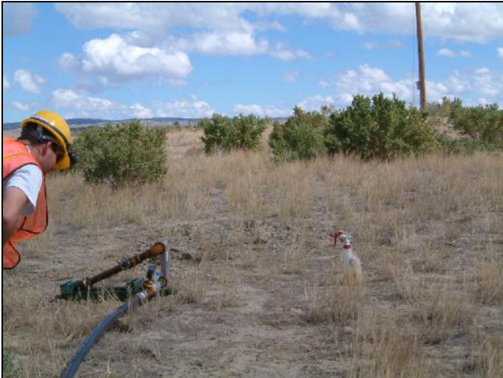
Site P3 – View of leak site and vegetation. The gas leak emits near the middle of the greasewood bushes.
