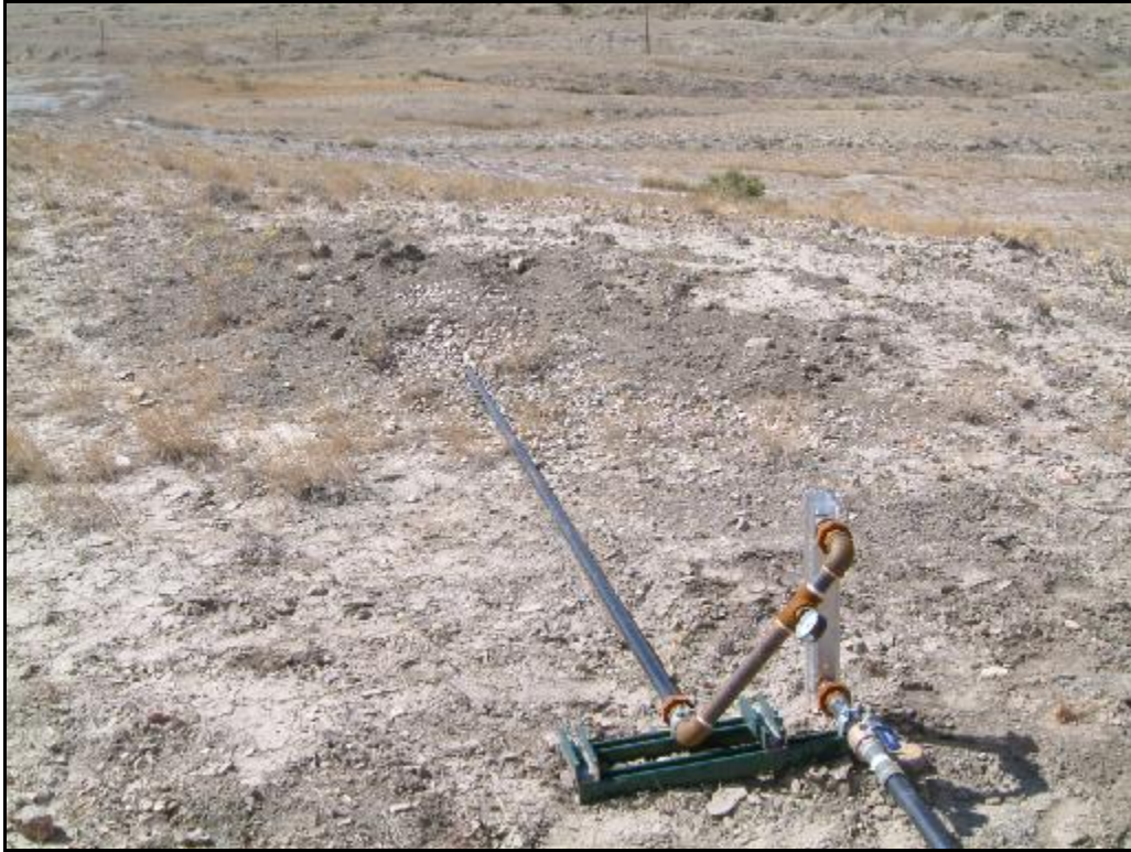
Site 6 – View at the top of the hill. Underground leak at gravel located approximately 10 feet from the rotometer.
