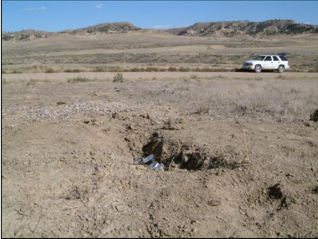
Site 2A – View from leak site to road. Underground leak located in the gravel area approximately 8 feet from bottle location.
