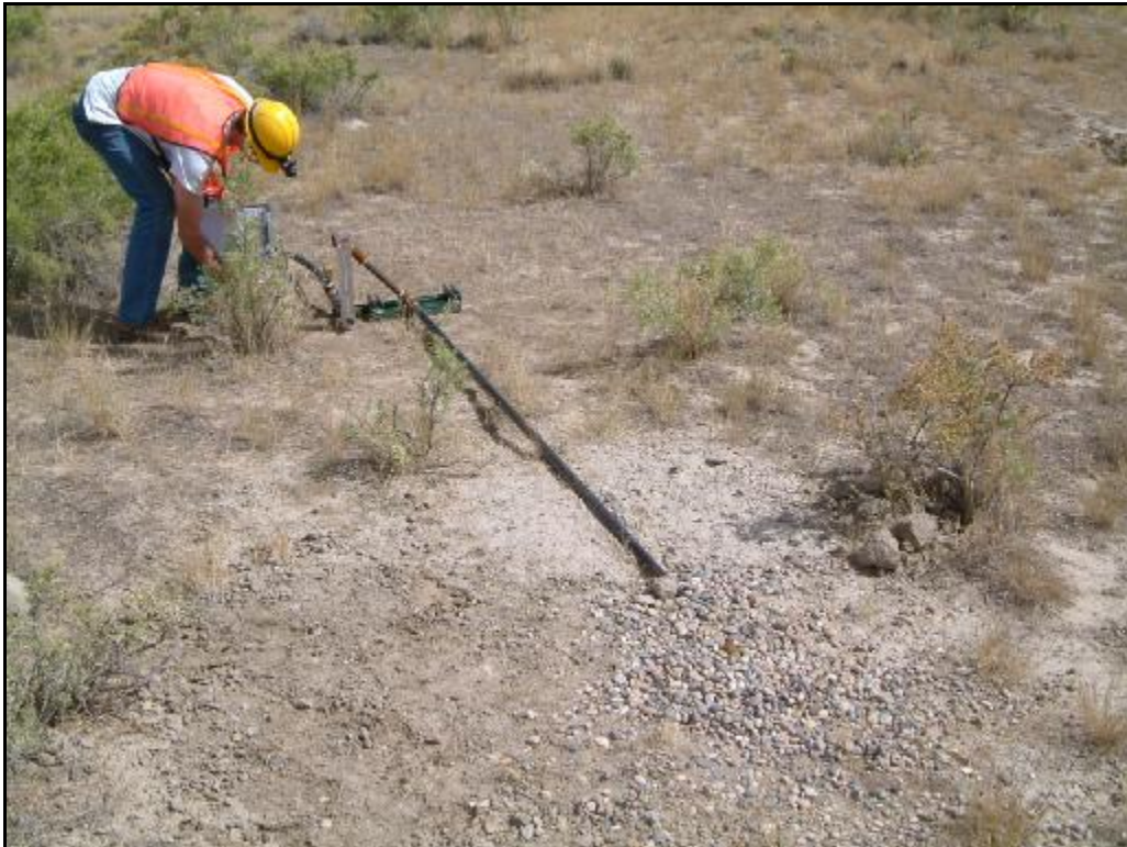
Site 4 – Underground leak emitting through gravel.
