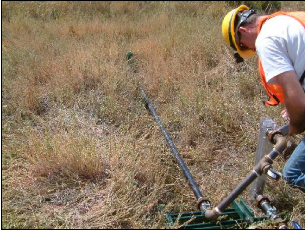
Site 3 – Aboveground leak at the end of the 10-foot long pipe.
