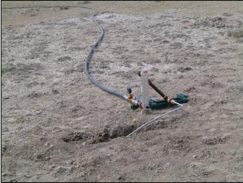
Site P1 – Detail of tubing entering the ground.
