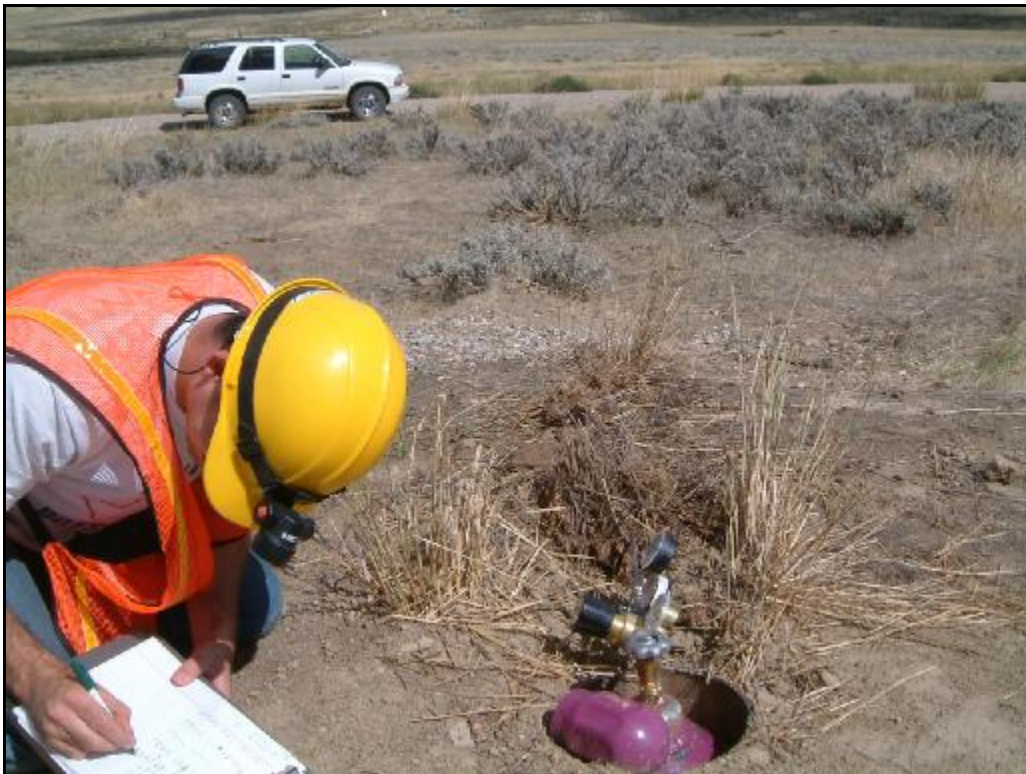
Site 2B – Underground leak located in the gravel area approximately 8 feet from bottle location.
