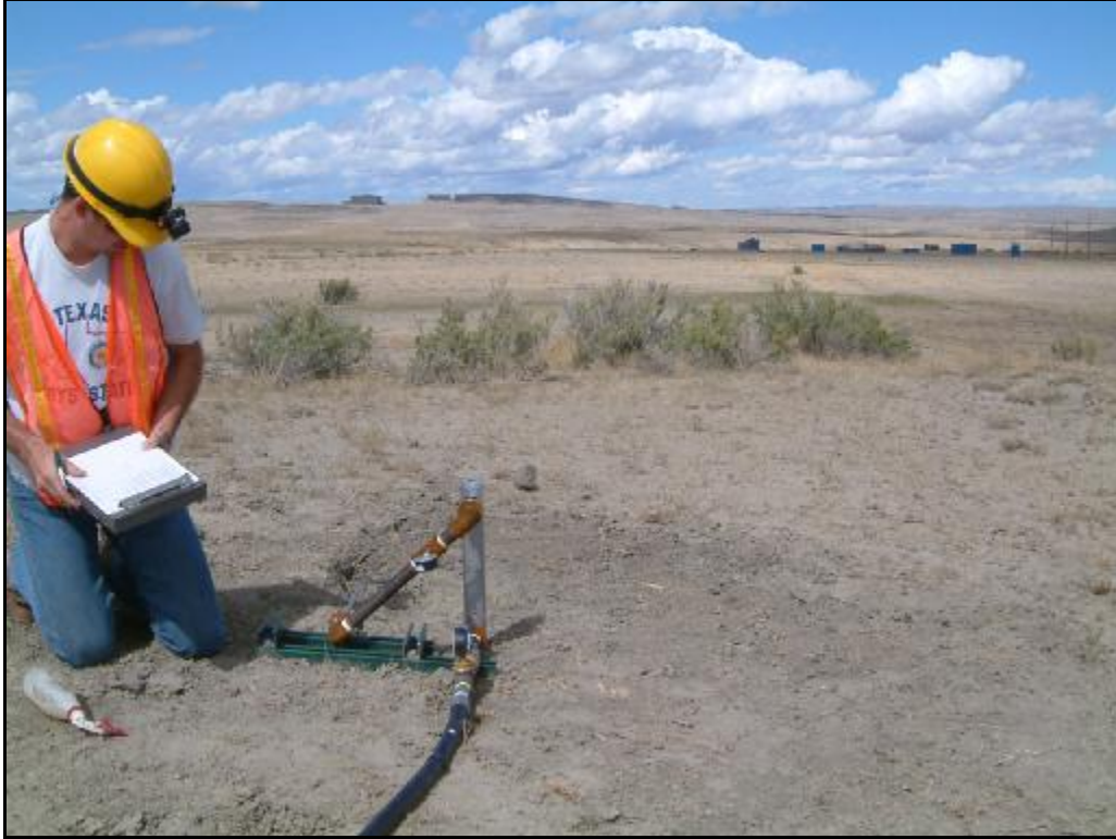
Site P2 – View of leak site and vegetation. The gas leak emits underground near the middle of the greasewood bushes.
