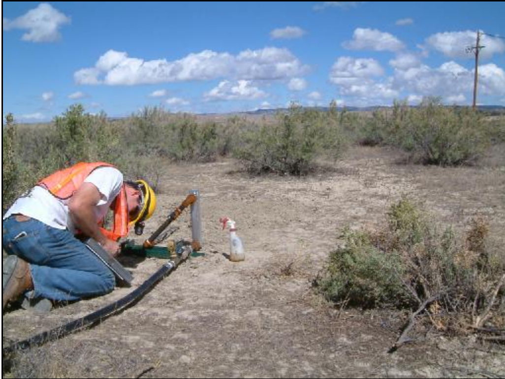
Site P4– View of leak site and vegetation. The gas leak emits near the middle of the greasewood bushes in the center of the picture.
