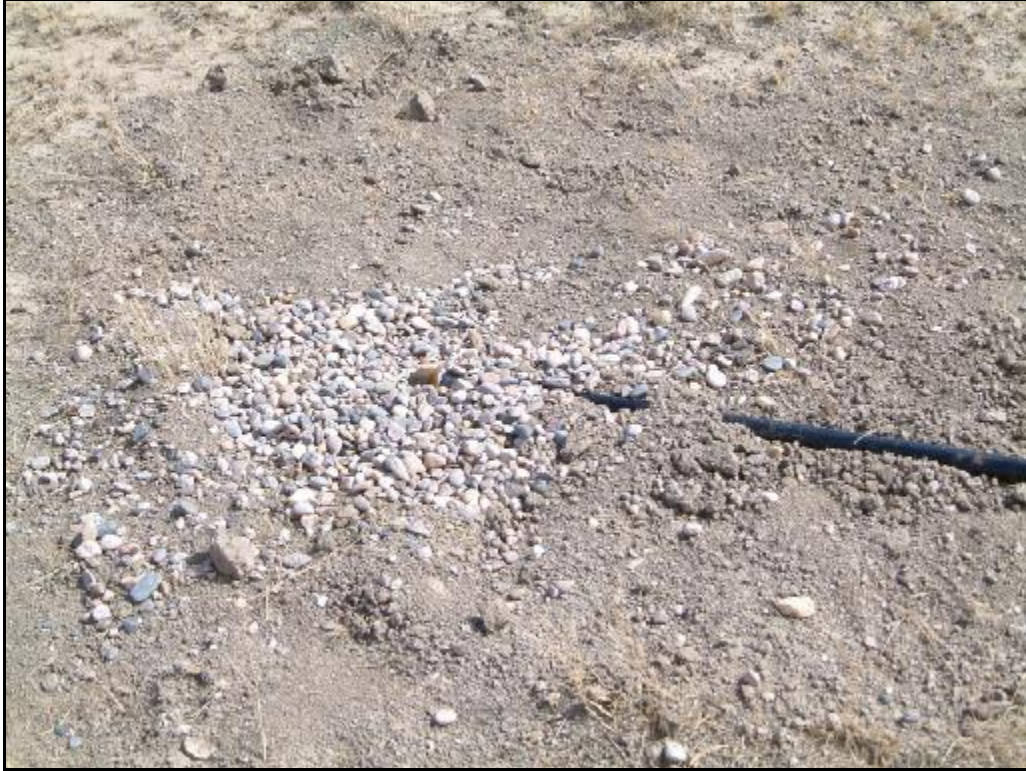
Site 5 – Detail of pipe entering the ground in the gravel area.
