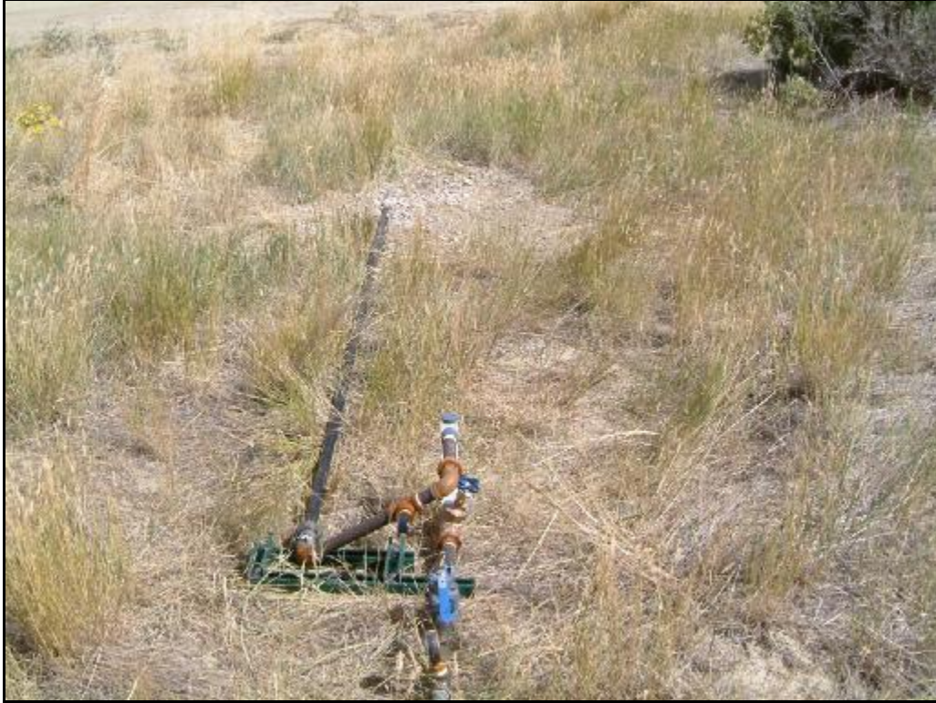
Site 1 – Underground leak outlet is roughly 10 feet from rotometer location (in gravel area).
