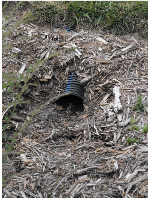
(Fig. 5) Buried downspout entering rain garden #2 showing channelization.
