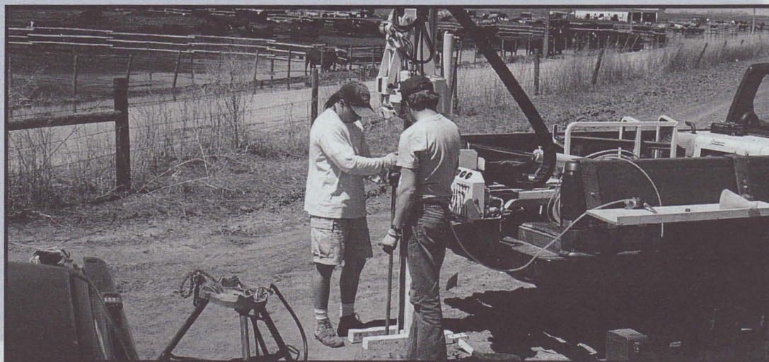
Data manager Pat Larsen and research technician Jeff Toavs install a groundwater monitoring well near a livestock operation in south central Nebraska. Monitoring for groundwater contamination around livestock confinement facilities is a project of NUs Water Sciences Laboratory (photo: Mark Burbach)
