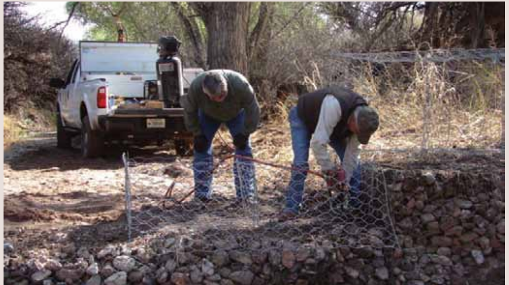
Volunteer Humberto Rodriguez (left) and heavy equipment operator Larry Brasher install wire gabions as part of an effort to restore native grasslands at San Bernardino National Wildlife Refuge, NM. (Chris Lohrengel/USFWS)
