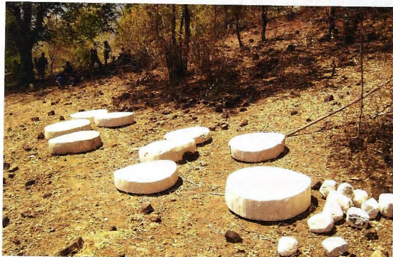
Fig. 7.4 Men and boys take a rest under the shade in the process of carrying the decorative stones to the original site on top-of the hill where Larigua is to be reconstructed.
