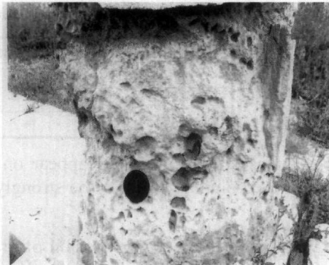
Figure 13 - Severe decay of bottom column piece constructed of type III sandstone and shape alteration
