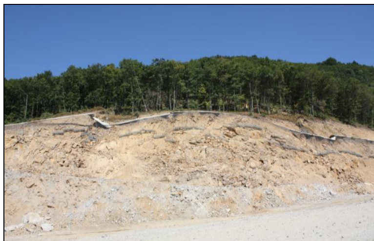
Figure 3 - The slide of the road cut O28. Drain trenches and benches have cracked.
