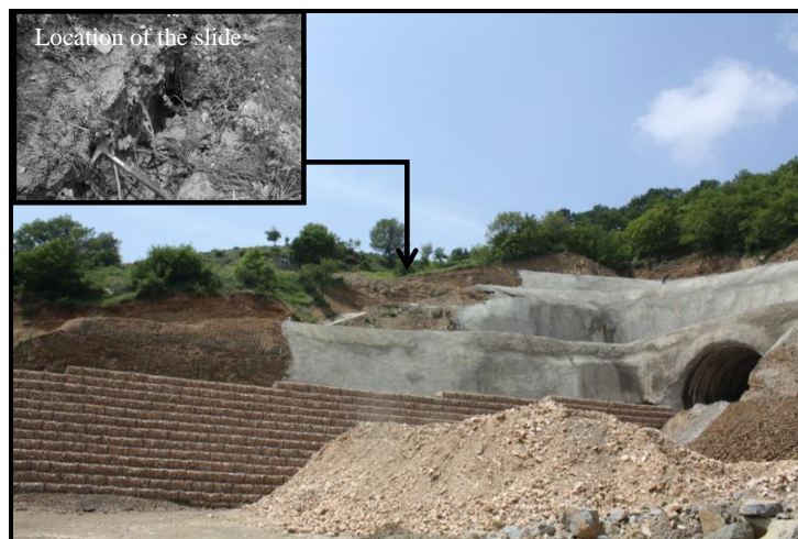
Figure 1 - View of the entrance portal of Nymfea tunnel. The gabion wall is used here for the stabilization of the whole slope. The slide occurred above the gabion wall.
