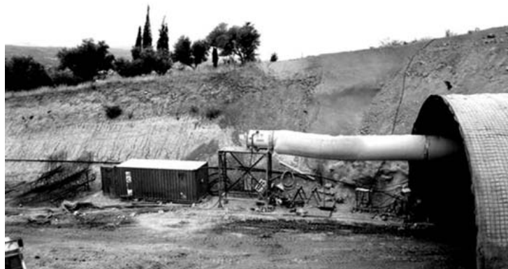
Photo 2: South part of Girokomion tunnel (Σ2), right branch. The Diluvial conglomerates cover with unconformity the Upper Geotechnical unit.
