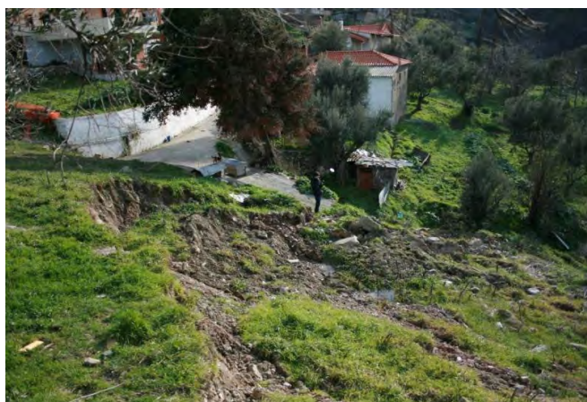
Figure 4 - Photo of the landslide taken from the northwest. Part of the small village road is collapsed.
