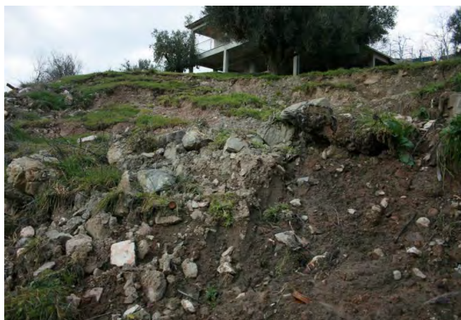
Figure 3. Photo of the landslide taken from the southeast. The head of the landslide is in front of two olive trees about two meters from the house basement.
