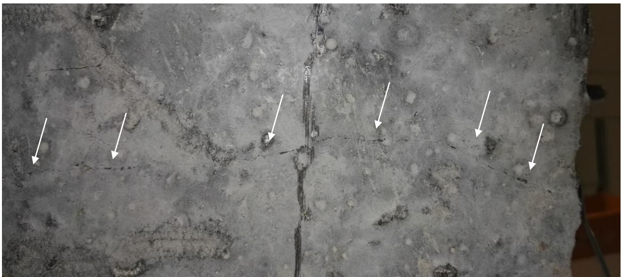
Figure 2.13. Crack developed under the sleeper. See Annex 1 for more photographs
