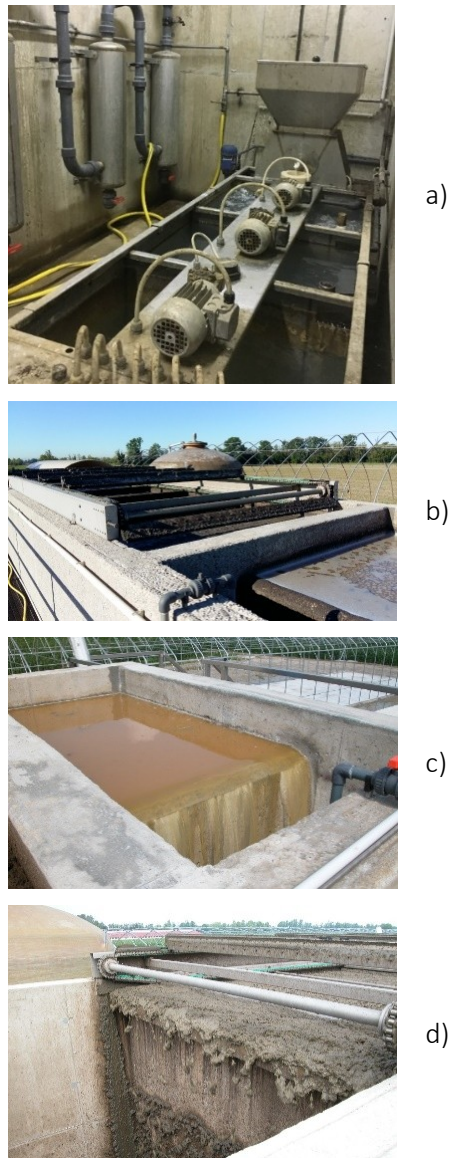
Figure 13 Floatation system of plant TP: a) chemical dosing, b) superficial chain scraper, c) liquid fraction obtained and d) the “solid” fraction obtained.
