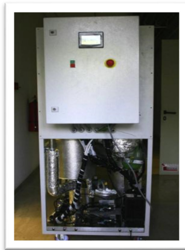
Figure 1.24. GH2-BE-5000 unit installed c/o the Dept. of Chemistry of Università degli Studi di Milano, for heat and power cogeneration.
