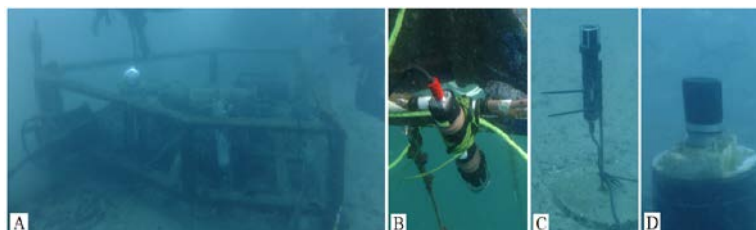
Figure 2. A) The OBSEA platform with its junction box and cable. B) Acoustic modem installed on the buoy. C) and D) are the acoustic modem and USBL, respectively, installed on the seafloor near OBSEA.
