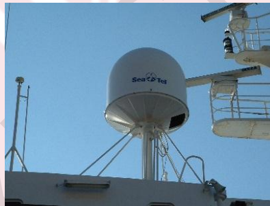
Figure 1.4: The shipboard radome installation. [Adapted from: (Croatia, 2015)]
