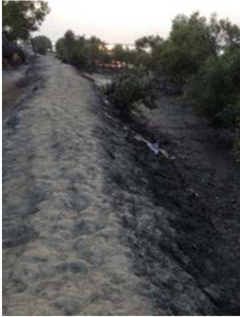
Fig. 06 A mud embankment or 'bandh,' Bali Island, Sundarbans.. Megnaa Mehtta Soon 3,500 kilometers of island peripheries will be replaced by concrete, cement and cinder blocks.
