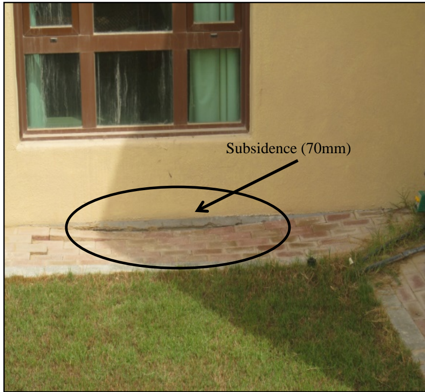
1 Subsidence of hard landscape adjacent to a villa
