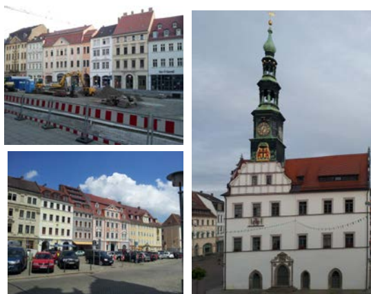
Figure 1. Façade restoration work in the German cities of Zittau (upper left), Görlitz (lower left), and Pirna (right)
