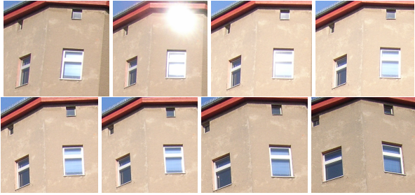
Figure 1. Eight different views of four windows of one façade. While the colour of pixels showing the surrounding masonry only changes slightly, the brightness of pixels of the window panes can vary a lot, especially when specular reflections occur.
