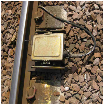
Figure 2.2.: An electro-mechanical treadle on the UK railway (Signalhead, 2009)
