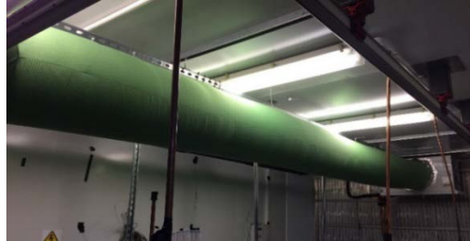
Fig. 2. Experimental test facility with air distribution via a round fabric duct.
