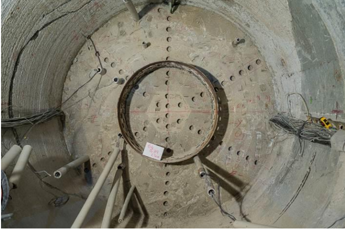
Figure 6. State of the barrier in the final dismantling. The location of the samples extracted from this section can be noted.
